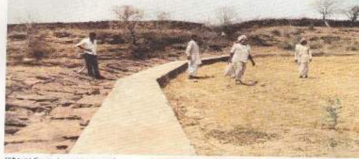
(Above) Concrete pagara, a soil conservation structure, built next to Kuchcha pagara in a village.
