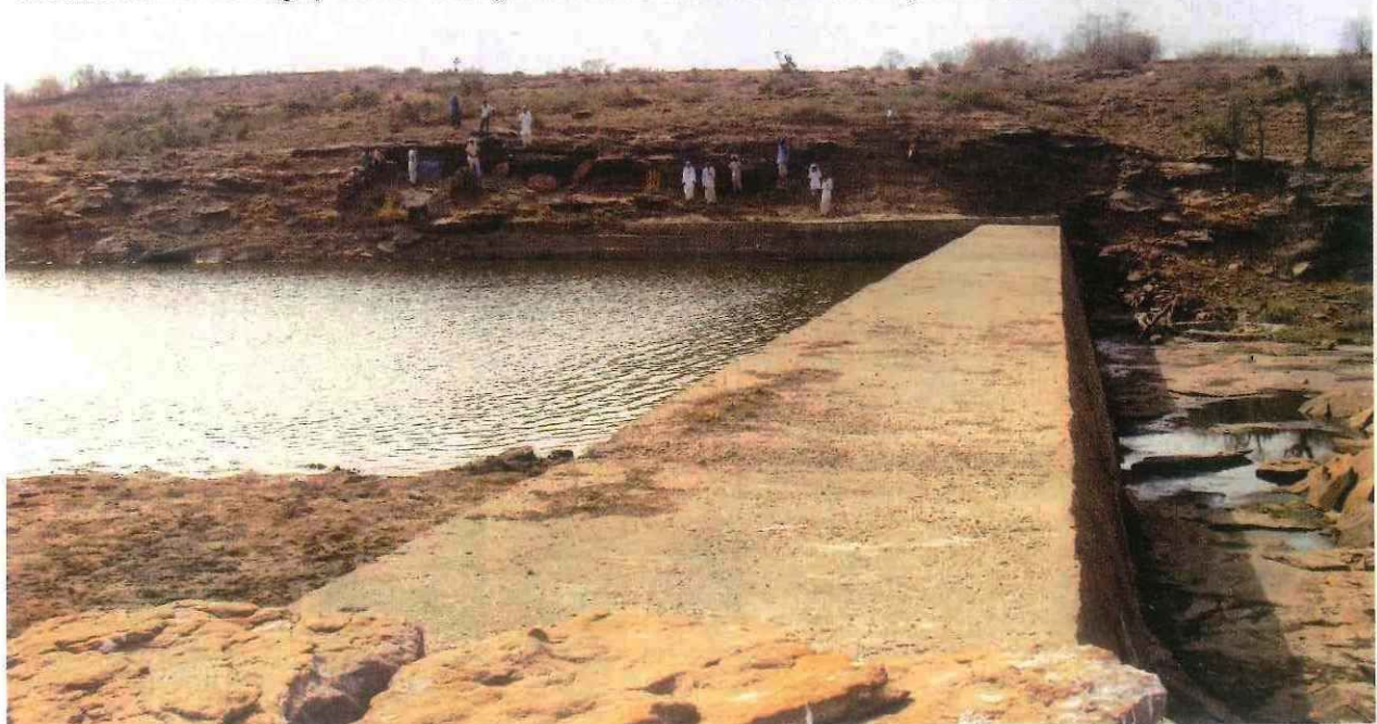
The anicut in Baraki village provides drinking water to cattle from at least six villages in Karauli district
